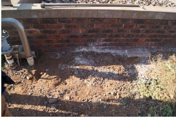
Spillages next to the drying bed (as shown by white powder)
