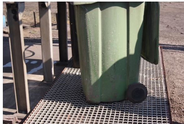
Containment system underneath drums
