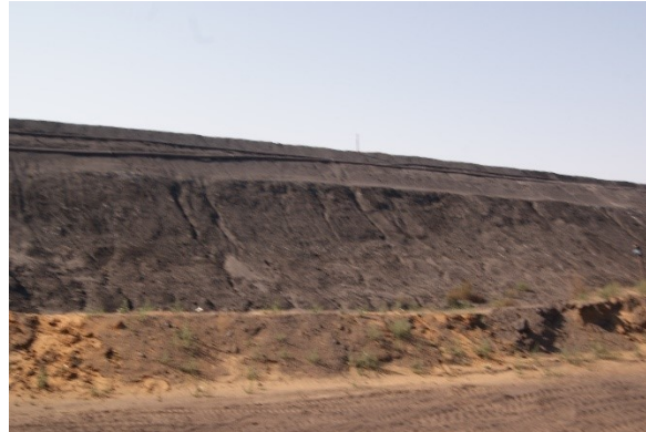
Old slimes dam's steep slopes
