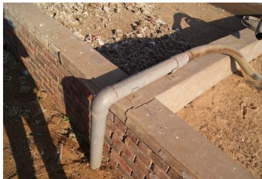
Cracked drying bed wall
