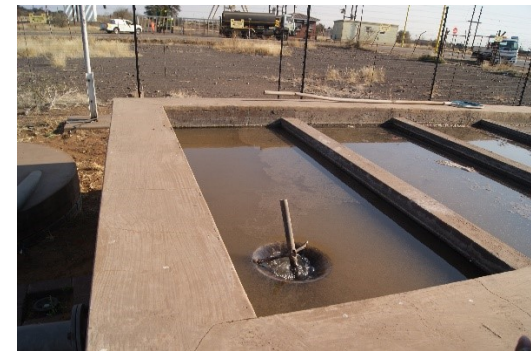
Chlorinator treatment not working
