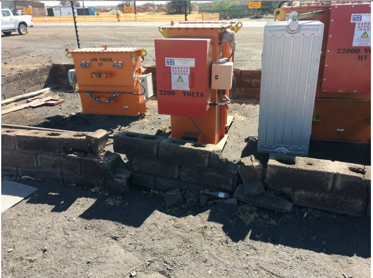
Figure 6.12: Example of defective bunds at Gloria Workshop
