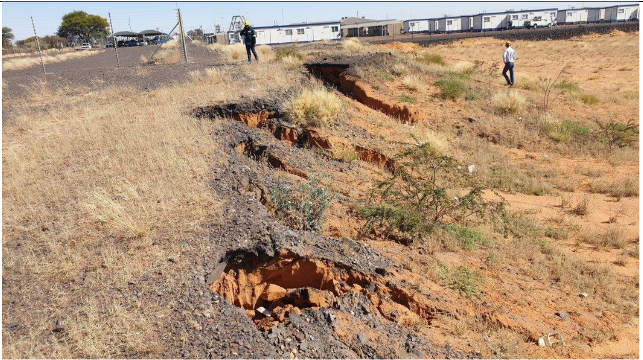
Figure 6.4: Erosion outside Gloria contractor camp
