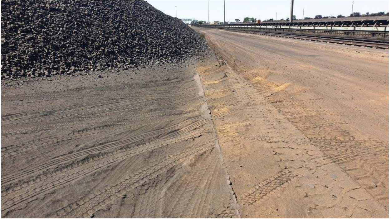
Figure 6.14: Stacker-reclaimer stormwater drains blocked.
