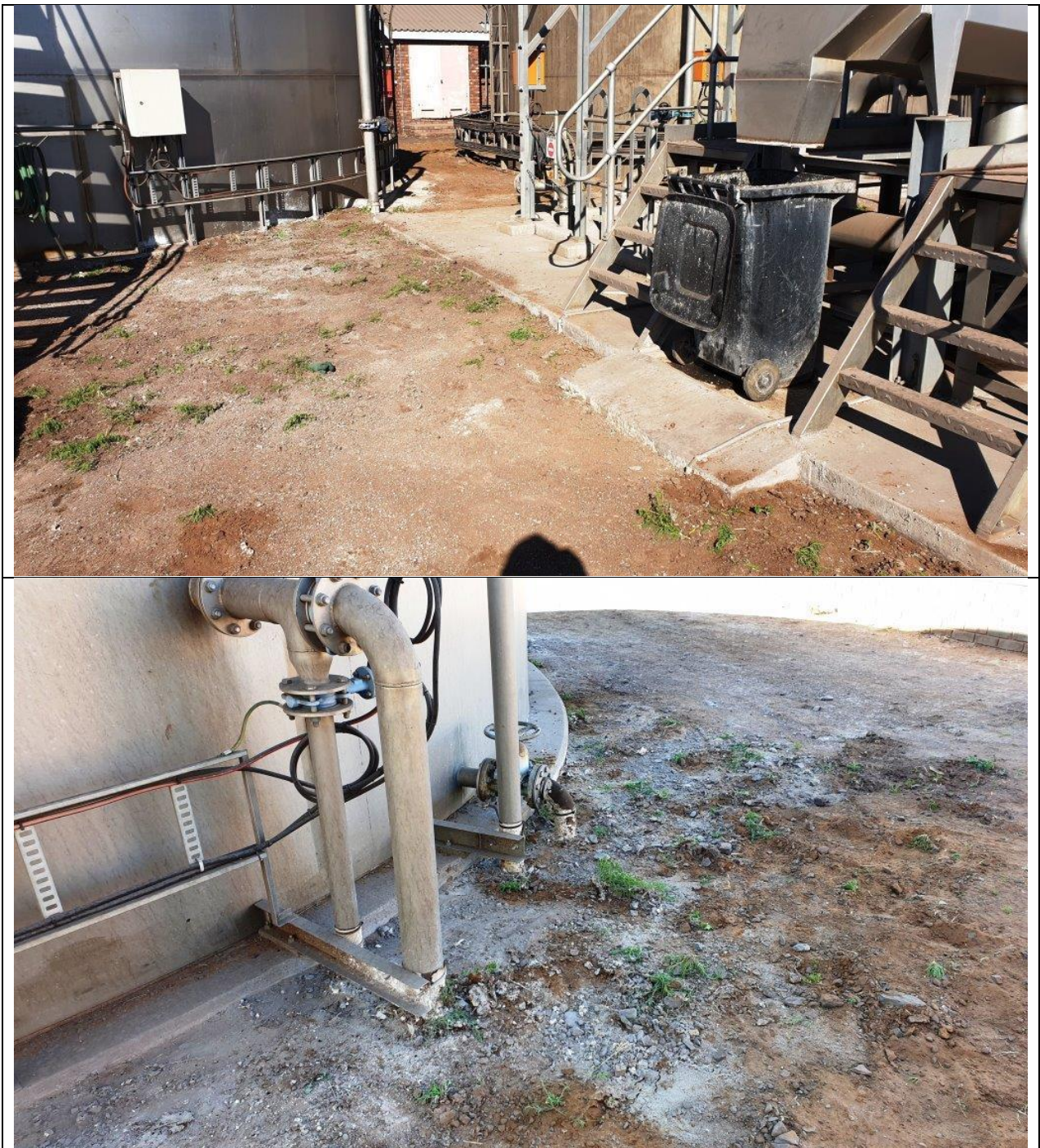
Figure 6.10: Overflows from at Gloria Sewage Treatment Plant
