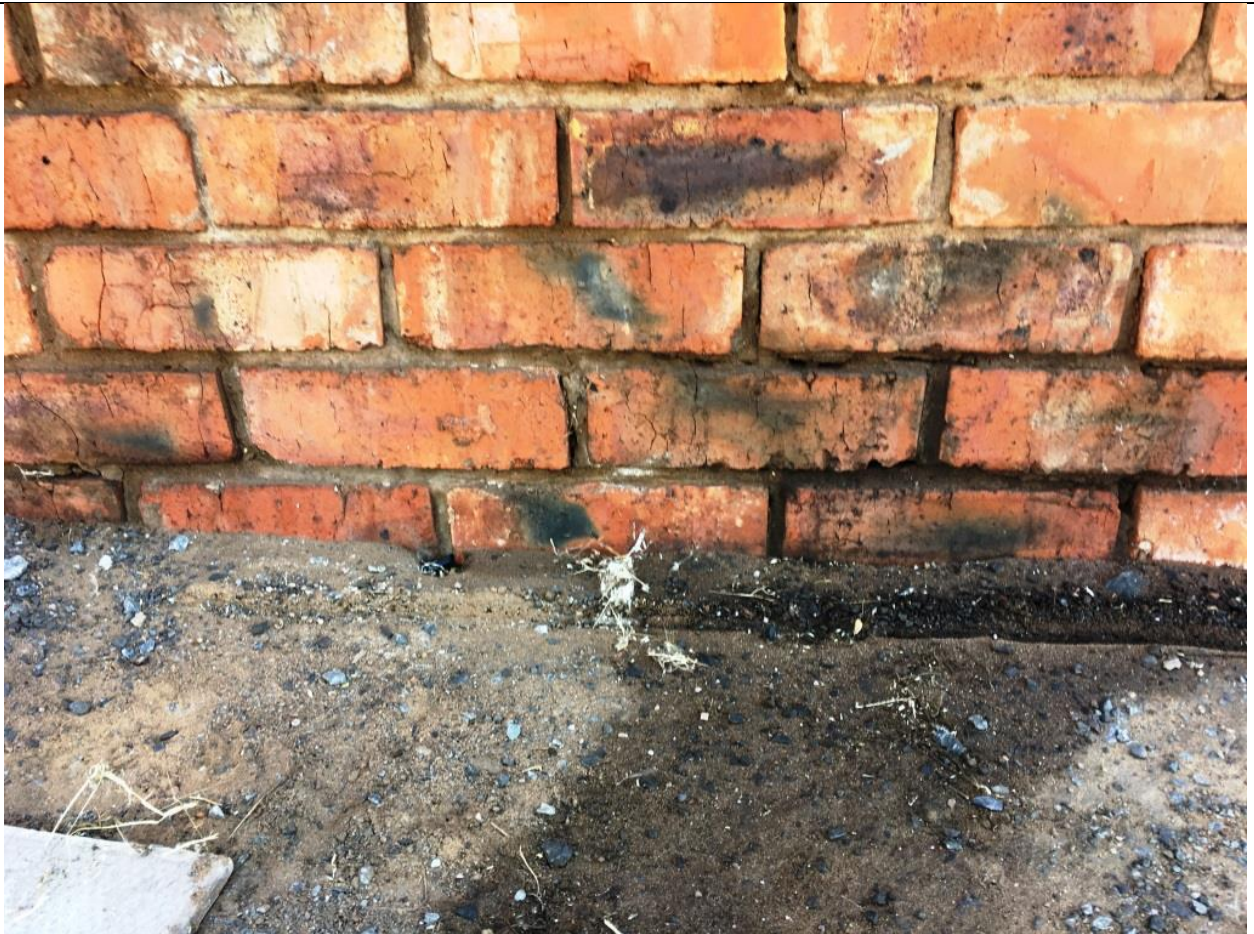
Figure 6.6: Leak emanating from the bund at Black Rock Hazardous Waste Transfer Station
